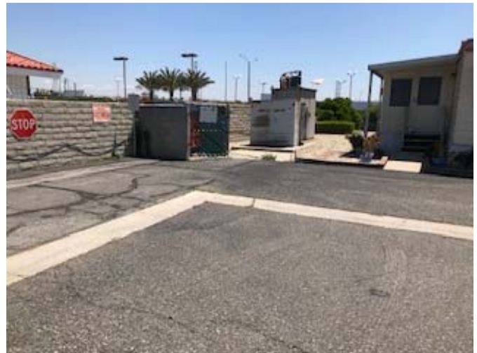
4. View of a trash enclosure and pad mounted transformer at the northeast corner of the Site.
